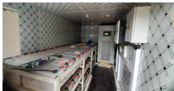
Figure 10: Salle des machines (batteries)
